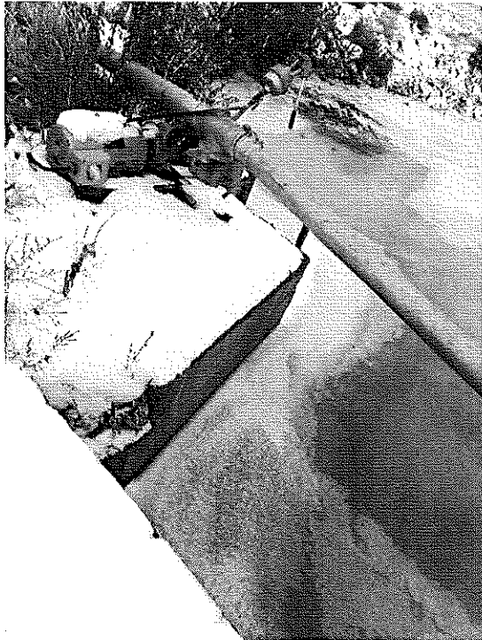
Photograph 4 Pump and impounded water on the upstream side of the diversion structure.
